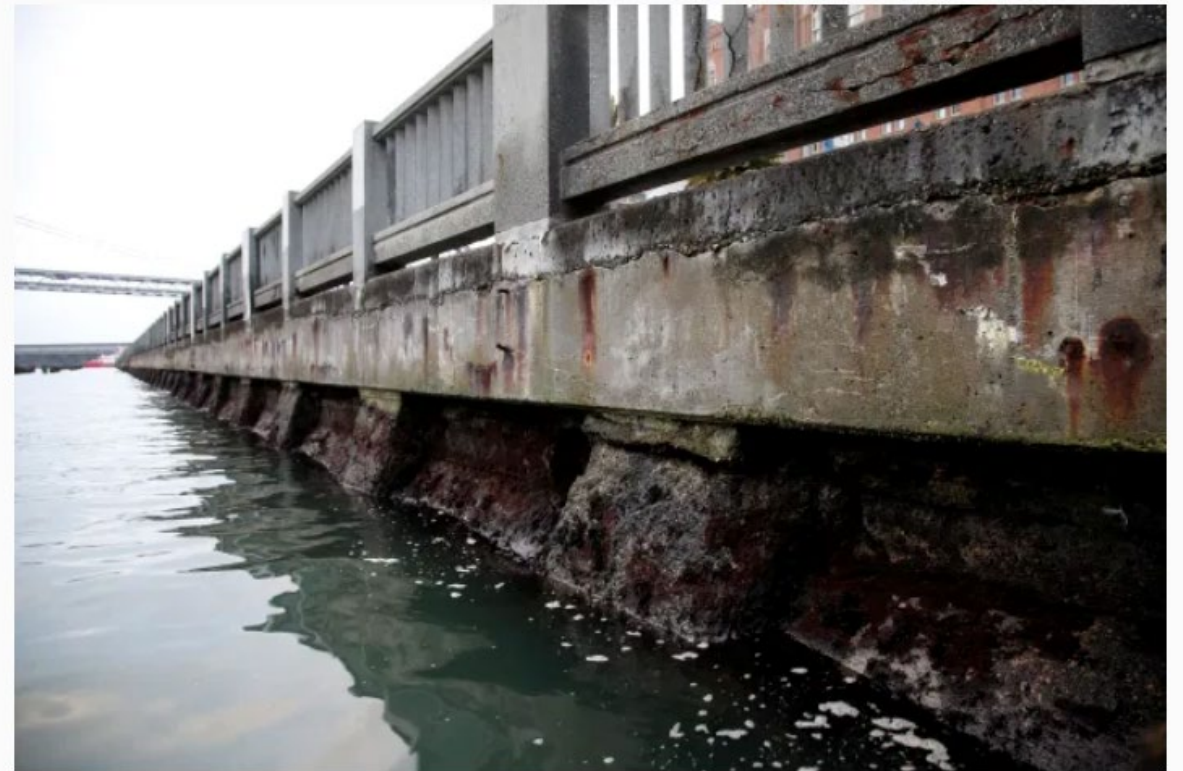
The crumbling sea wall in San Francisco is the subject of Proposition A, a $425 million plan to rebuild the 100-year-old structure that runs the Embarcadero from Fisherman's Wharf to the San Francisco Giants ballpark. (Karl Mondon/Bay Area News Group)
