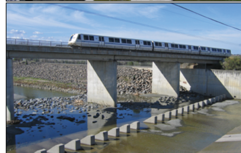
In 2006 the San Francisco PUC removed Sunol and Niles (pictured) dams from Alameda Creek, alleviating public safety concerns and providing steelhead and other fishes' access to upstream waters. The flood control channel downstream (BART photo) still presents various obstacles to fish. Photos by Brian Sak.
